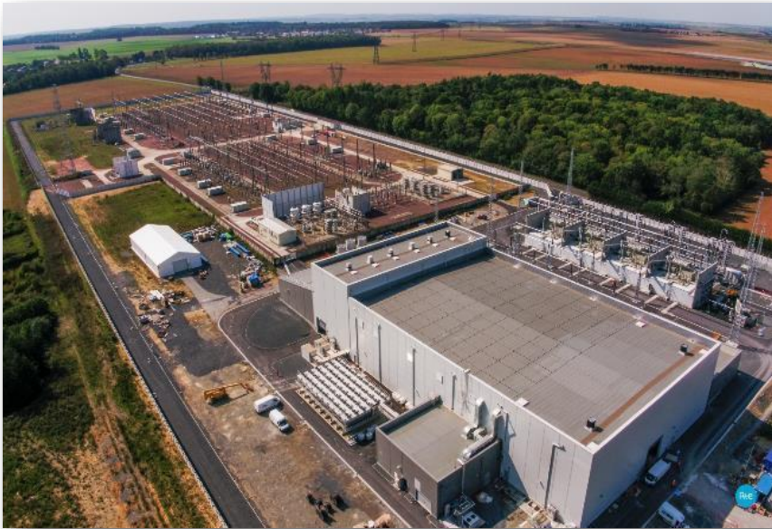
Station de conversion HVDC 320 kV – 5 ha (et poste de raccordement) – 13 ha RTE - IFA2
